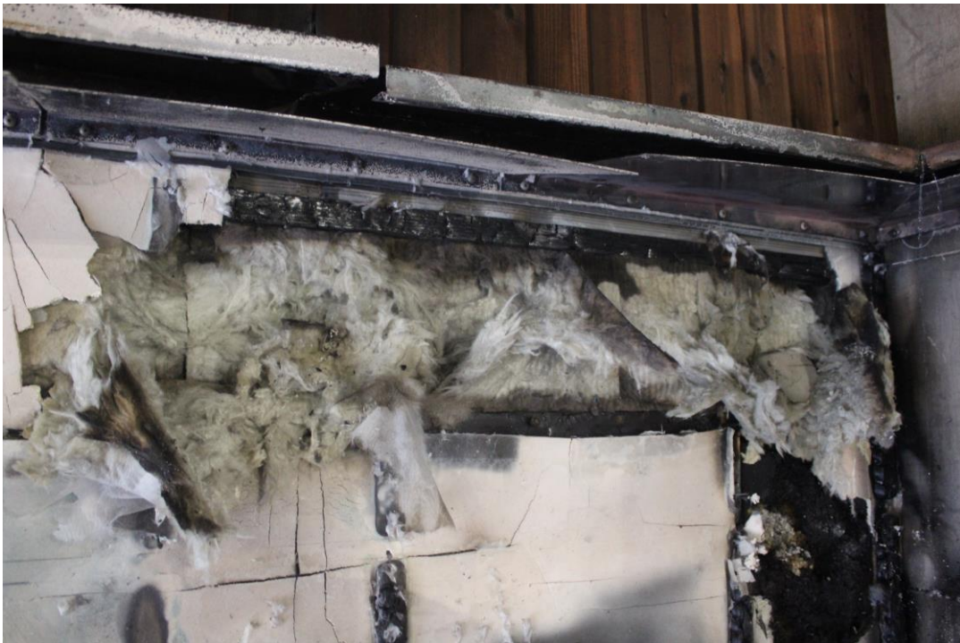
Photo No. 26 Test specimen after the test. Corner below the second flame deflector after removing weatherboard.
